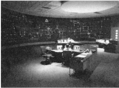
FIGURE 67.1 Central dispatch operation arena of Entergy Corporation’s Beaumont Control Center (Beaumont, Texas) which includes a modern EMS.
