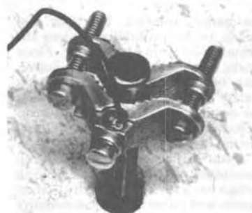
Figure 7. Typical static control ground connection
