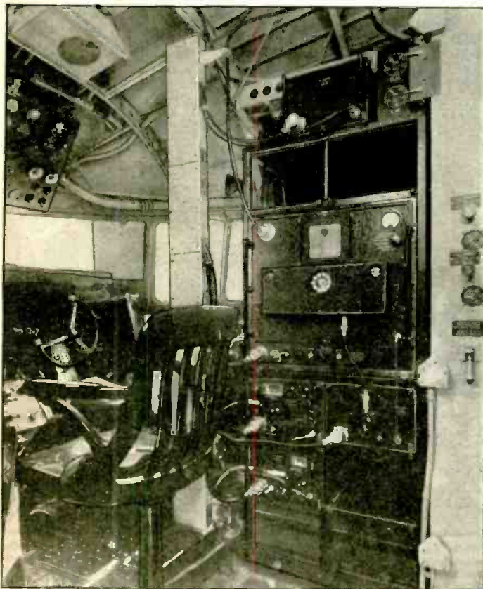
Eleven units of radio equipment will ultimately guide the giant DC-4; only 5 are shown here. The radio rack holds (top) the inter-communicating system amplifier; (next lower) the 250-watt transmitter joined through flexible shafting to the communications receiver below it. The auxiliary receiver is seen immediately to the left of the latter unit and below it is the beacon receiver. When aloft, radio operation is governed remotely by a control column.
