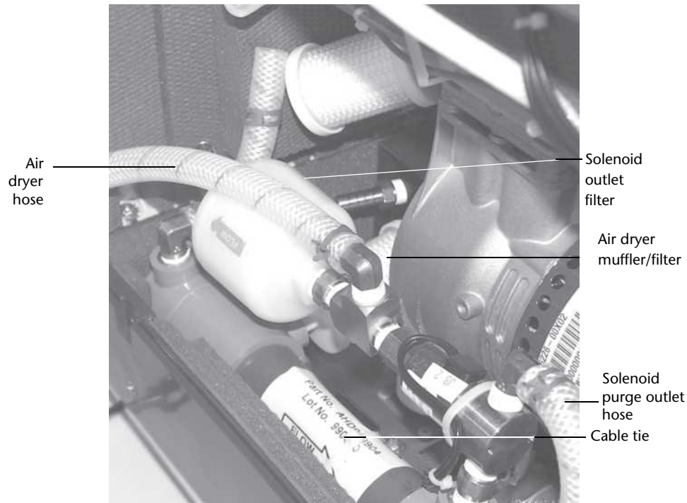
Figure 8-99. Air dryer/solenoid valve assemblies installed
