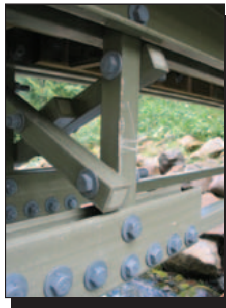
Figure 31—This truss was damaged by dragging or improper handling.
