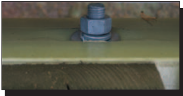
Figure 32—The bottom chord was damaged by dynamic loads from ATV traffic, by bolts that were overtightened, or by overloading.
