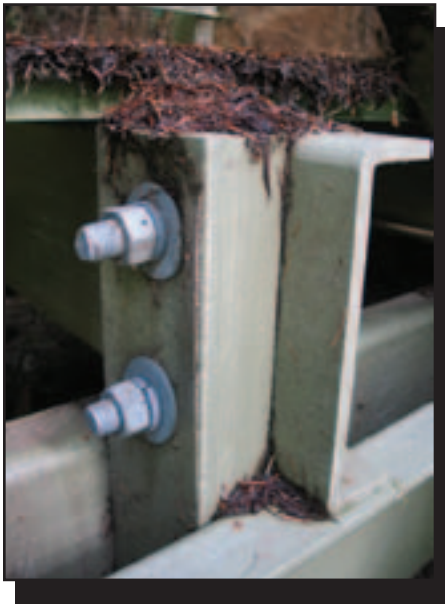
Figure 43—This floor beam tie was damaged when bolts were overtightened.
