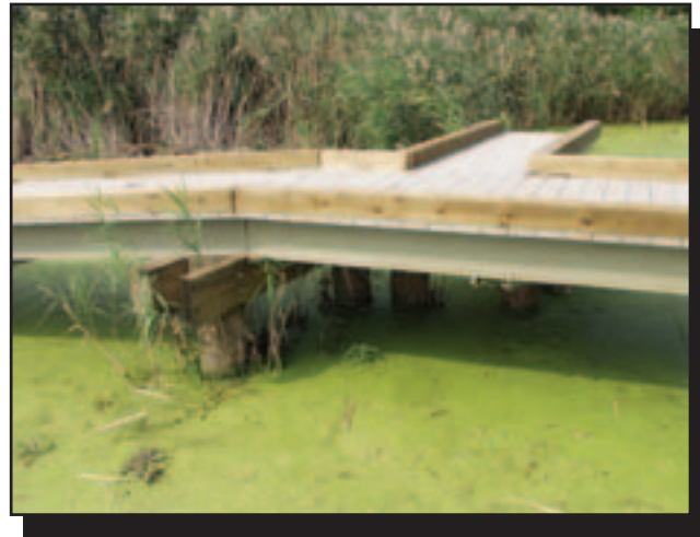
Figure 6—This boardwalk on Staten Island was constructed using an FRP deck-beam system.—Courtesy of E.T. Technics, Inc.
