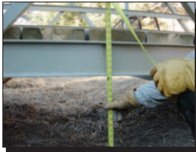
Figure 24—A tape measure can be used to check a bridge's camber and deflection.
