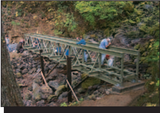
Figure 38—Installing one of the tested FRP bridges at Falls Creek in the Gifford Pinchot National Forest.
