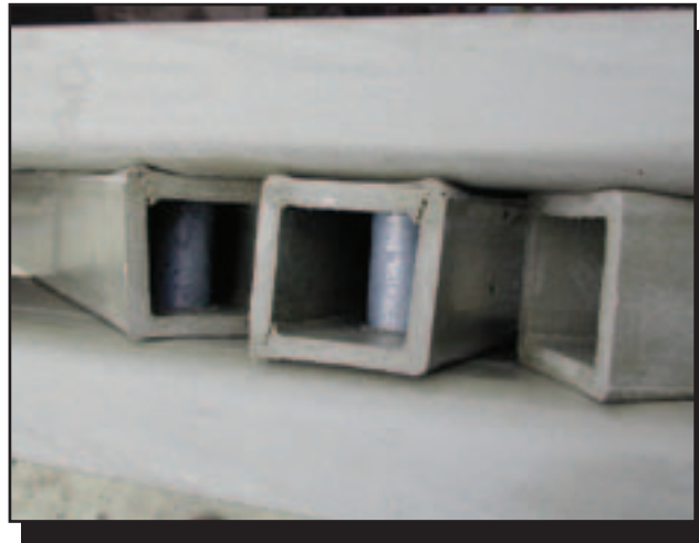
Figure 23—Overtightening bolts cracked two tubes.
