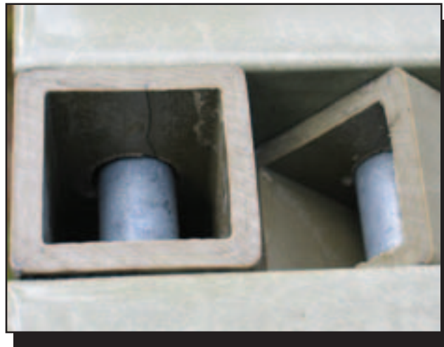
Figure 45—This joint at the top of a vertical post was damaged when bolts were overtightened.
