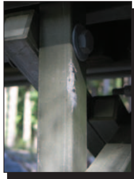
Figure 41—This truss was damaged when it was dragged or handled improperly.
