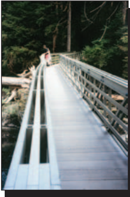
Figure 28—The top chord bowed on the left side truss of the Staircase Rapids Trail Bridge in the Olympic National Forest.
