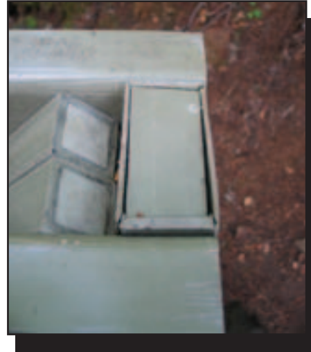
Figure 29—This joint at the top of a vertical post was damaged when bolts were overtightened. The material was thinner than the \frac{1}{4} inch minimum now recommended.
