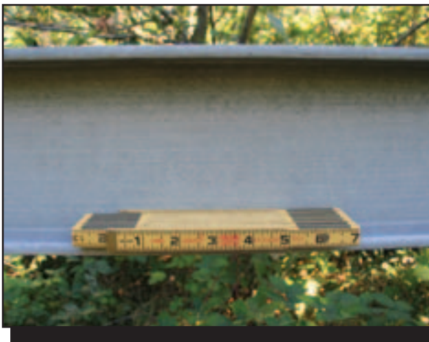
Figure 30—The lower section of this member of an FRP bridge is discolored because the coating that protected it from ultraviolet light wore off.
