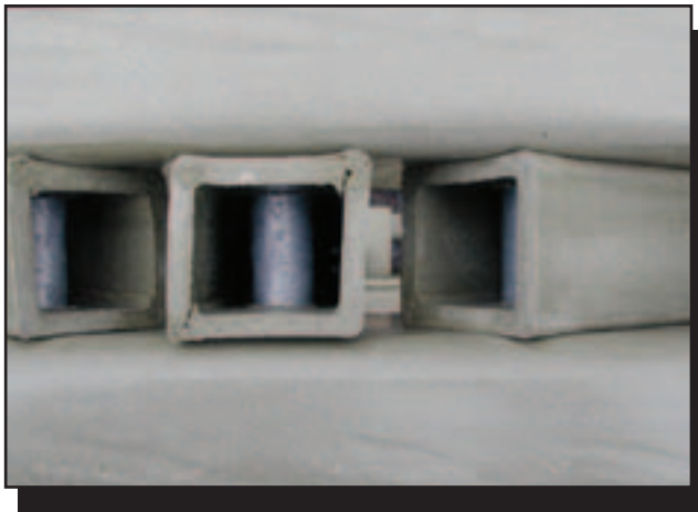
Figure 47— This joint at the top of a vertical post was damaged when bolts were overtightened.
