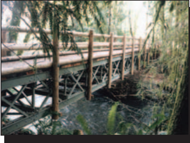
Figure 7—A deck-truss FRP bridge in Olympic National Park. This bridge uses FRP materials for the trusses and wood for the rails, maintaining a natural appearance for a high-tech structure.
