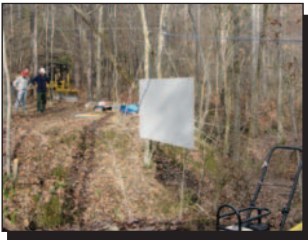
Figure 12—A skyline system can be used to haul bridge materials to an abutment across a stream.
