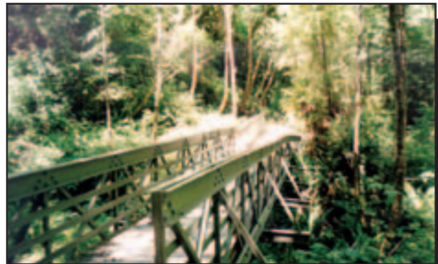
Figure 27—This FRP bridge in Redwood National Park began to fail when a loaded mule train was halfway across. No one was injured.
