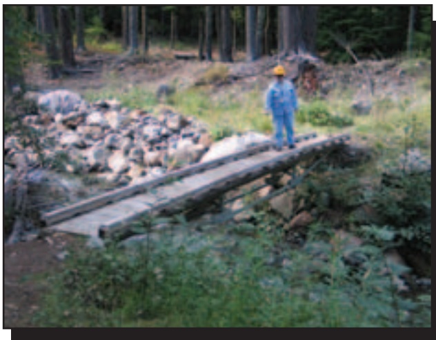
Figure 40—This deck-truss FRP bridge in the Mt. Hood National Forest has an inverted queen-post configuration.
