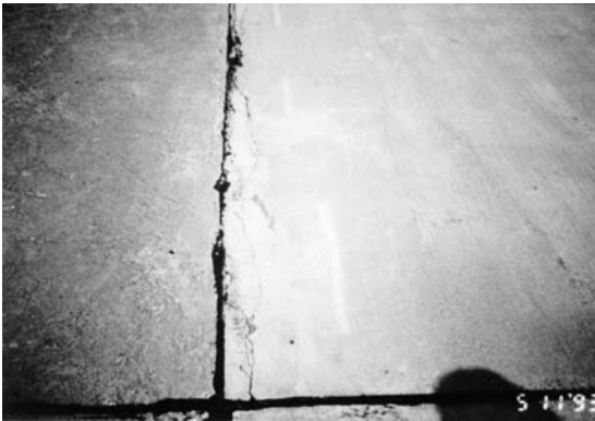
Figure 4.1. Moderate-severity spalling along an expansion joint
