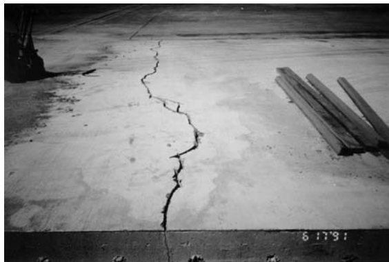
Figure 10.2. A freshly sawed crack
