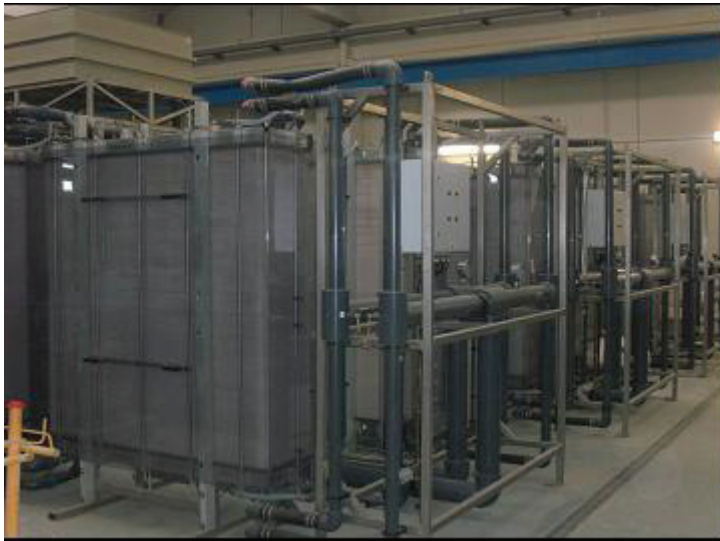
Fig. 4. EDR stacks at the Depurbaix WWTP.
