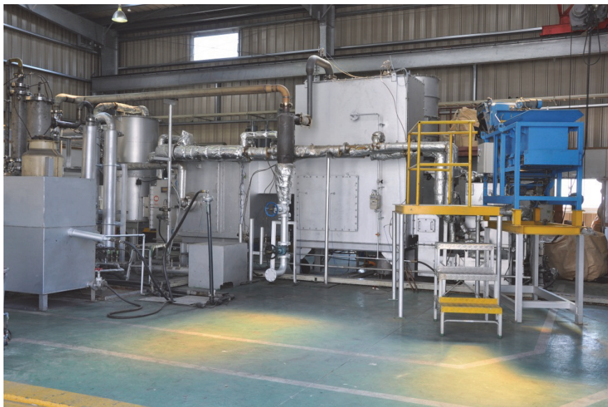
Fig. 9. "Norin Biomass No. 3" test plant located in Sakai Kougyo, Ltd., Isahaya City, Nagasaki, Japan.
