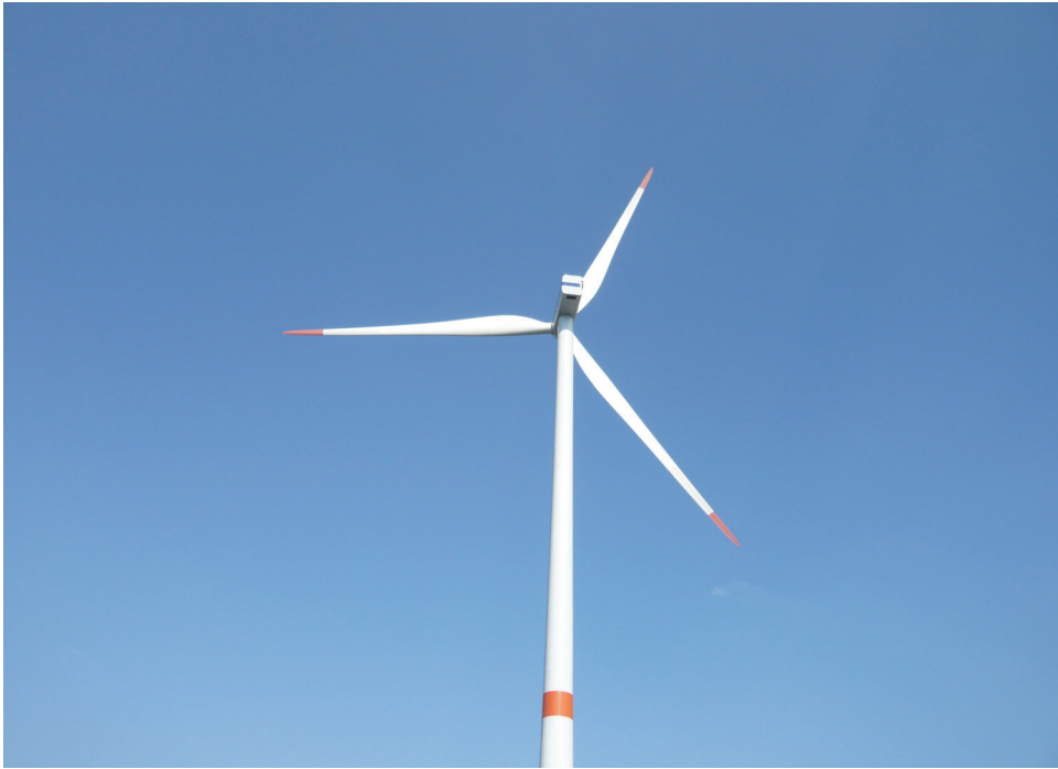
Fig. 4. View of a rotor blades, nacelle and upper section of the Vestas wind turbine tower
