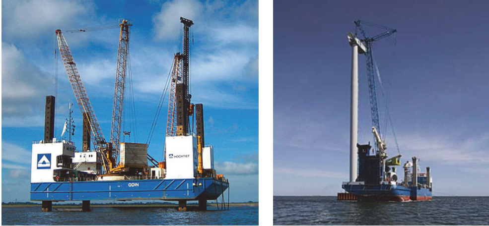
Fig. 5. Examples of external cranes for replacement of large components; Jack-up barge ODIN (left) and crane ship
