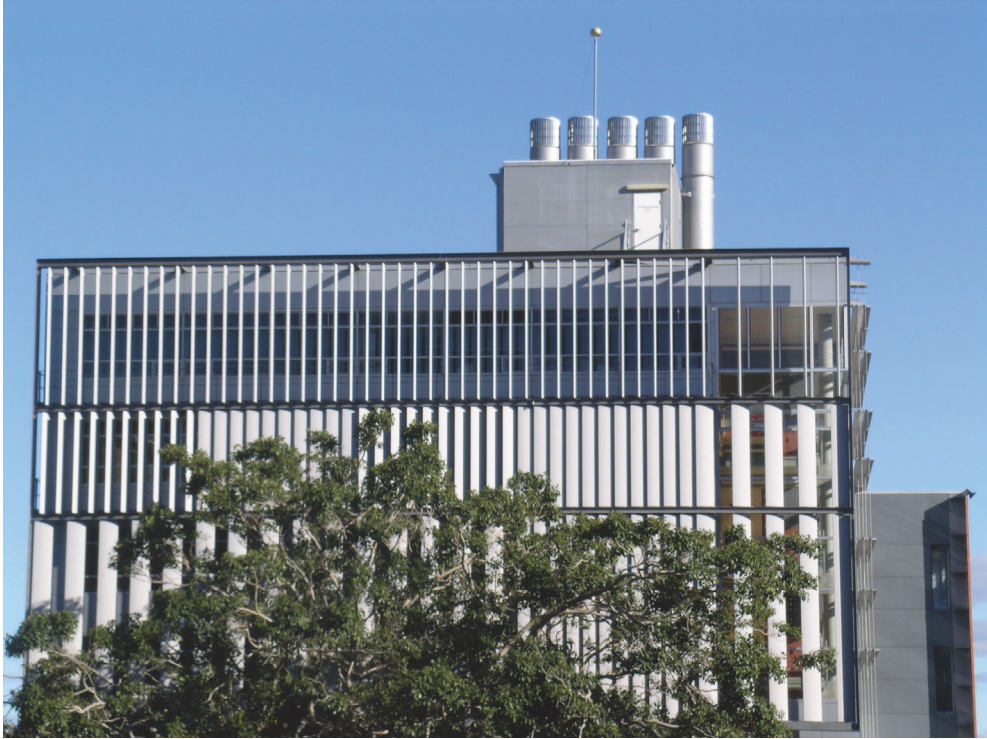
Fig. 16. Rotating ventilators in use on the roof top of building at the University of New South Wales
