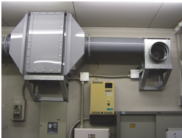
Fig. 6. Centrifugal blower (right), charcoal filter housing (left) and humidifier (center).
