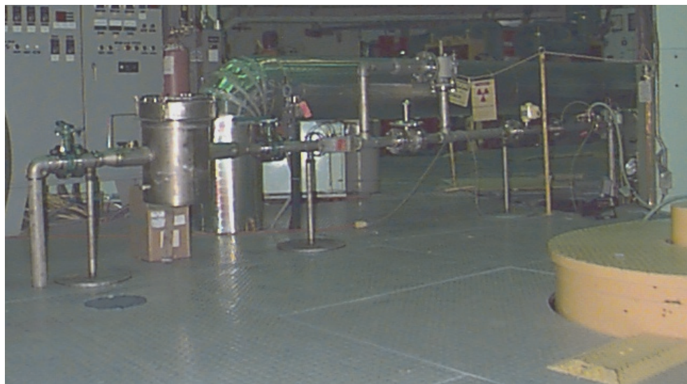
Fig. 8. Vent line for EBR-II Primary Tank with installed instrumentation and HEPA filter.
