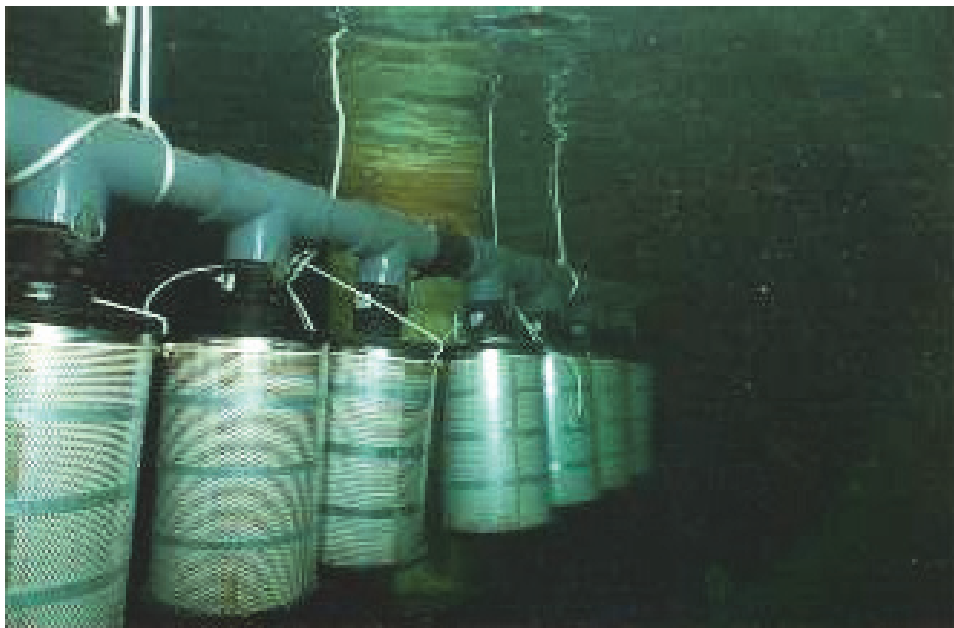
Fig. 4. UCC vacuuming filtration system underwater manifold.
