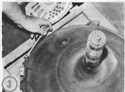
Tube is in the cabinet and the brackets are fastened down. The straps were carefully tightened on tube after brackets were attached to cabinet.
